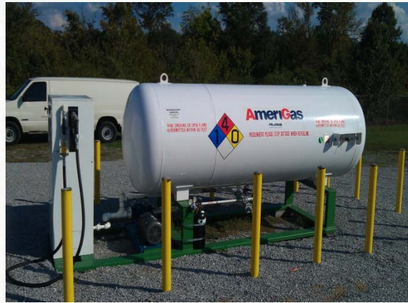
AmeriGas Propane Tank
